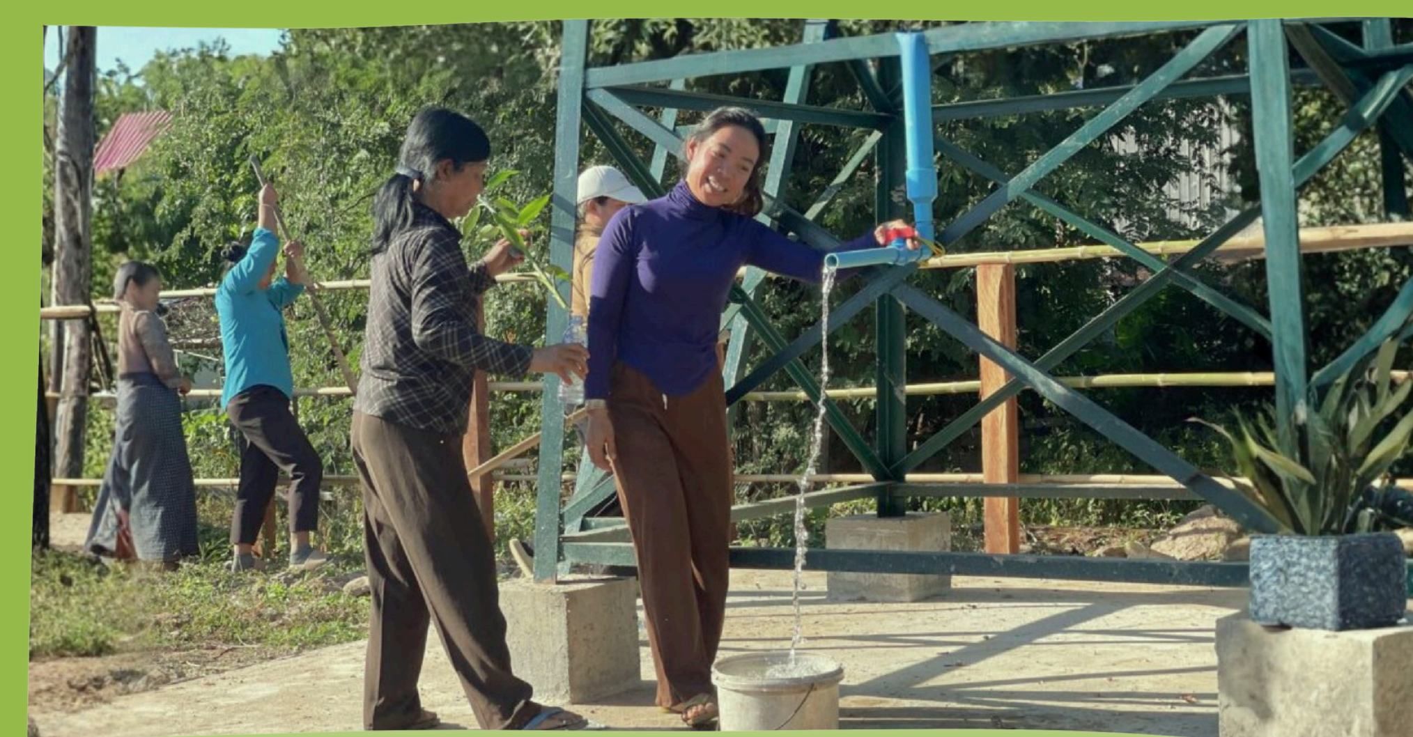
Solar water Pump in Koh Sneang village
