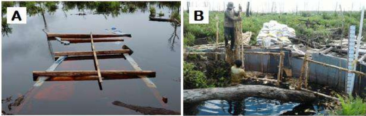
Figure 6 (a) Canal blocking was established during rainy season; (b) Construction of the canal blocking
